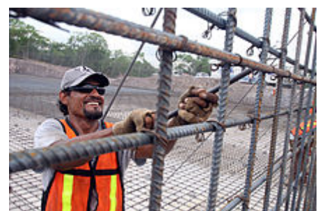
Worker assembling rebar for a water treatment plant in Mazatlan, Sinaloa, Mexico.
